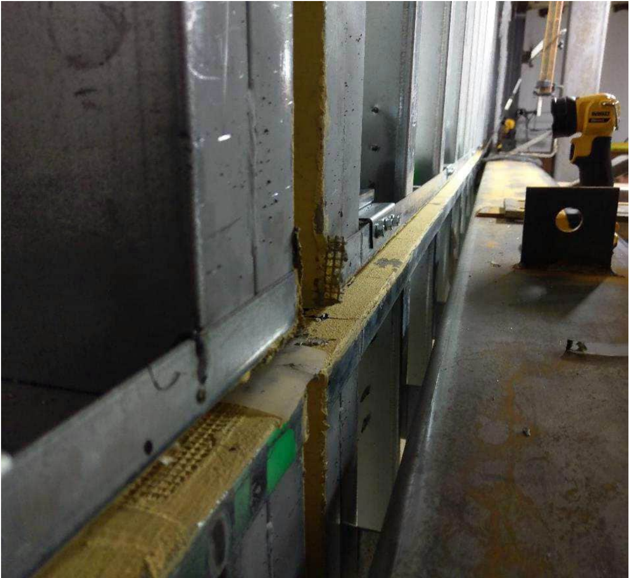
Photo B16: Interstory horizontal (in/out) movement test, 1.45" outwards
