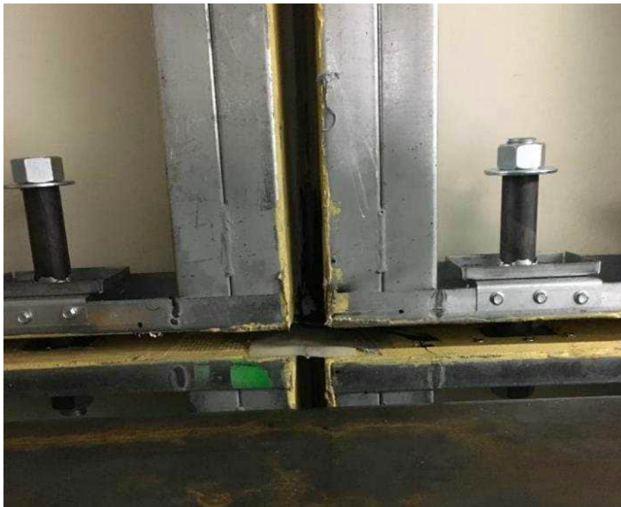
Photo B19: Interstory vertical (up/down) movement test, 0.75" downwards
