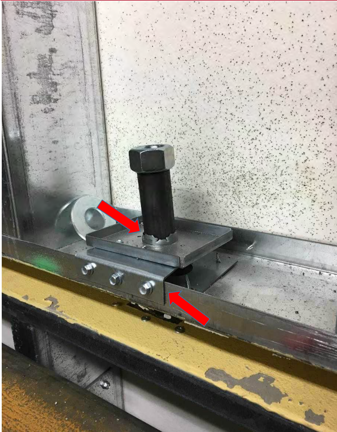
Photo B7: Remediation: Additional safety support brackets for each panel to panel sliding pin connection at the horizontal panel to panel joint. Fastened at each existing support bracket.
