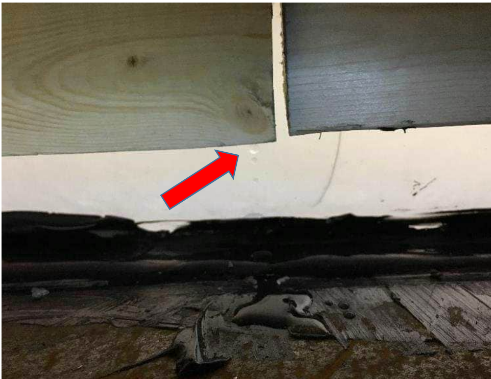
Photo B9: Water penetration over the sill at the mid span of the lower full size panel.
