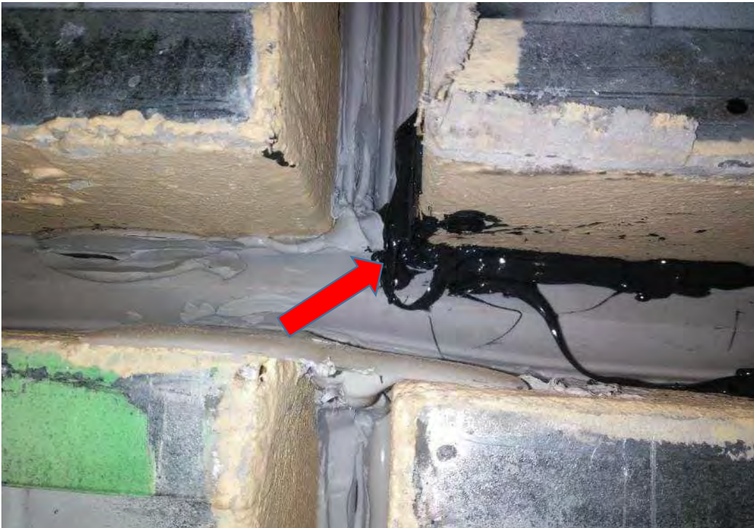
Photo B6: Remediation: Four-way joint was resealed with Dow 995 sealant from the interior side “Prior to section 2.1B, Preload”
