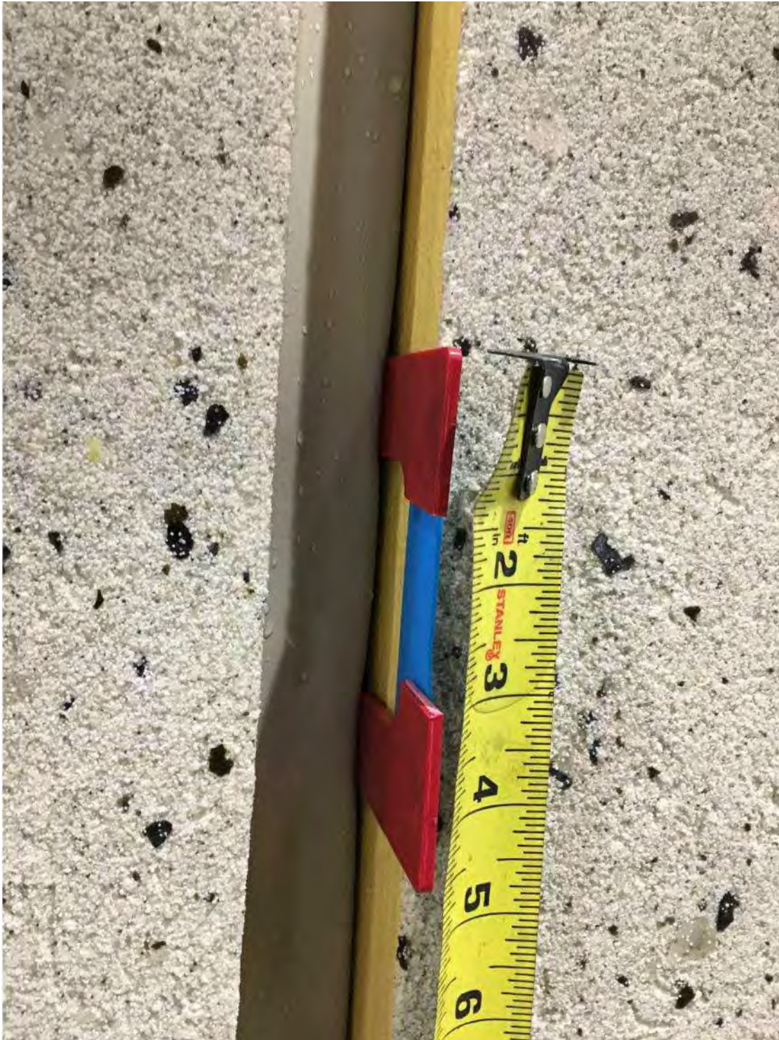
Photo B21: At 32 inches above the horizontal expansion joint two 1/8 inch shims were inserted into the vertical expansion joint seal at 4.5 inches apart to simulate a defective seal "Prior to section 2.14 Water Penetration Test "
