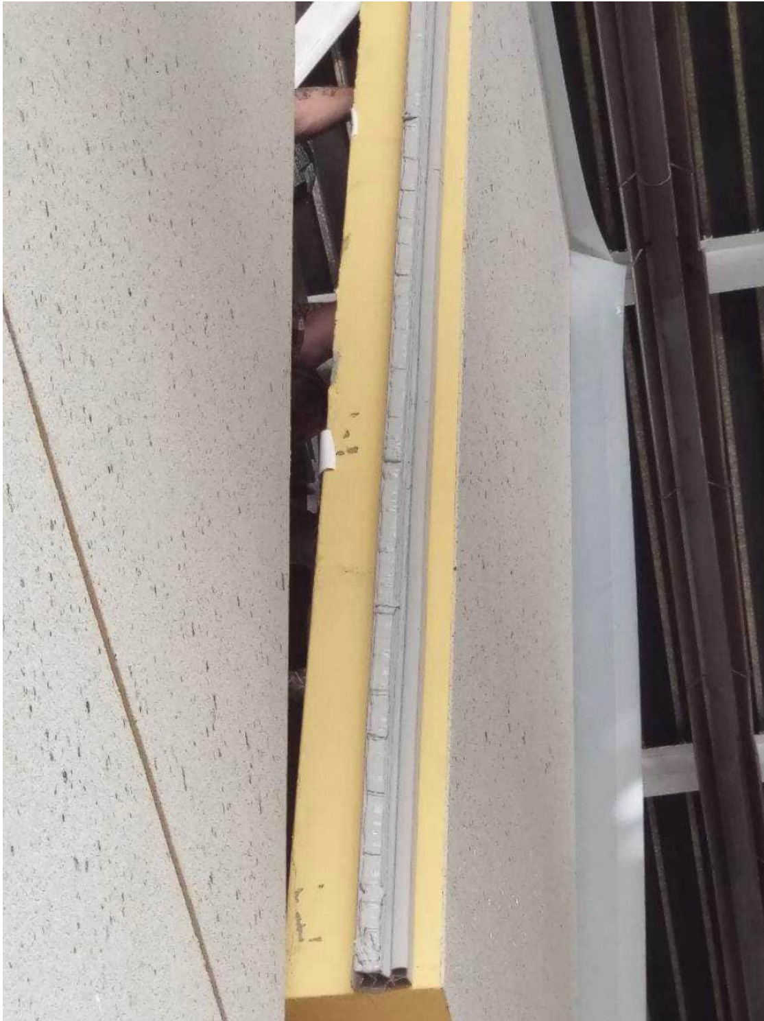
Photo A21: Final panel installation sealant application at vertical panel to panel joint
