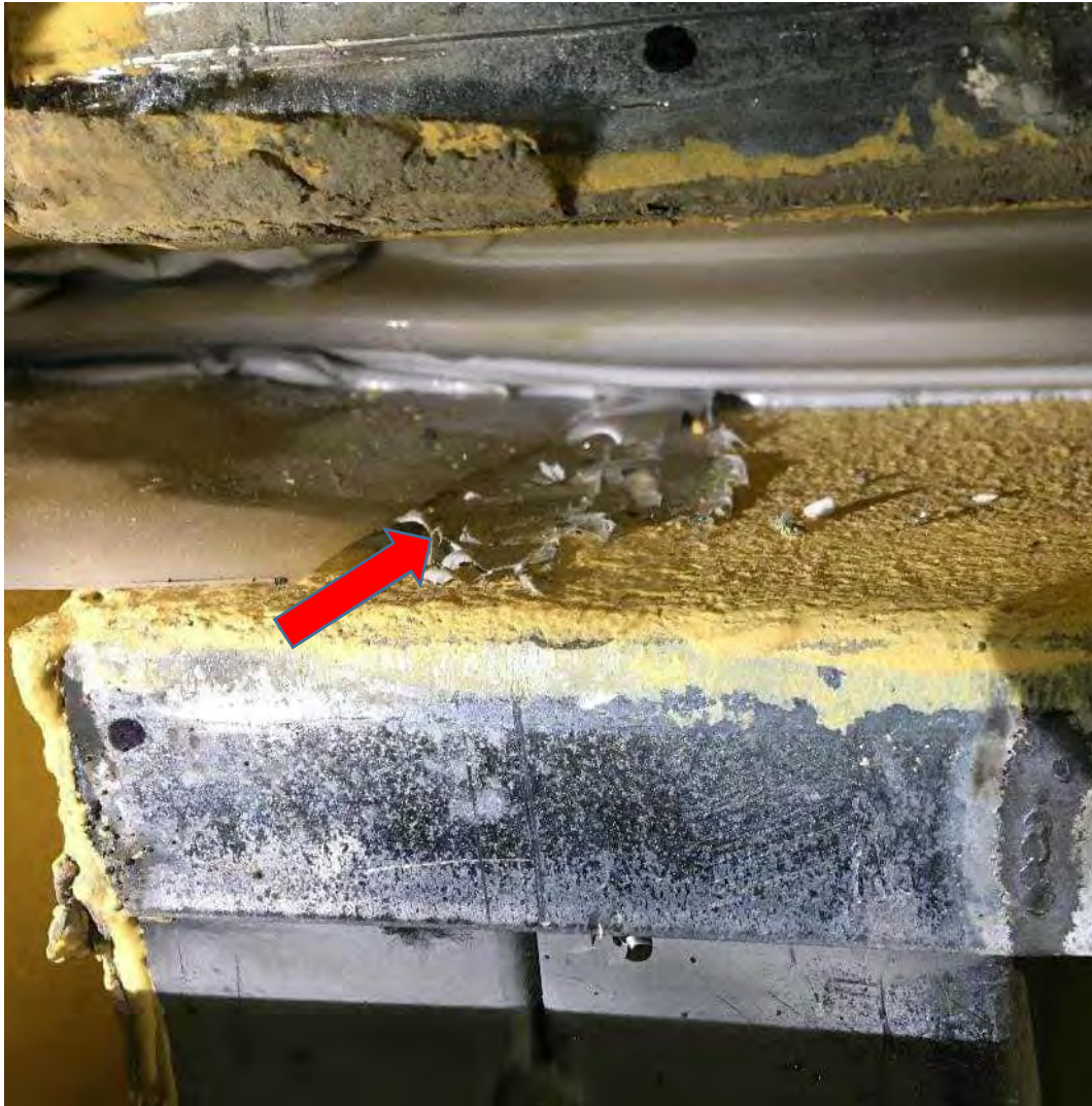
Photo B4: Water penetration through four-way joint during static water penetration test (Test procedure 2.3a).
