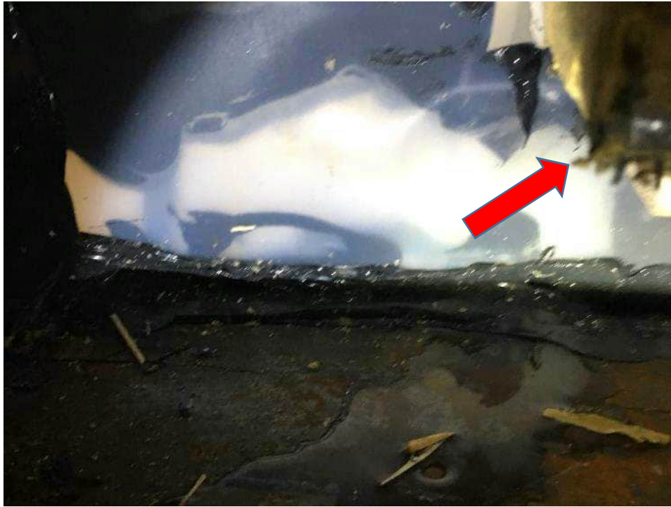
Photo B8: Water Leakage along the left (from exterior) transition membrane sealed joint.
