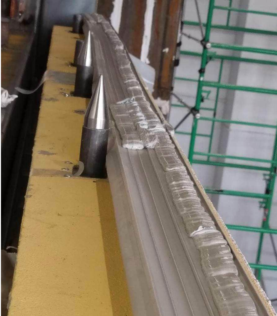
Photo A19: Guide pin installation at the horizontal panel to panel joint
